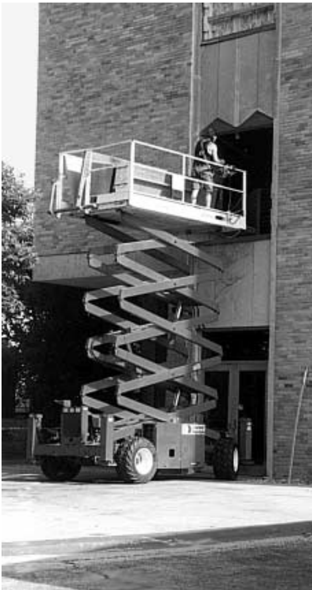
Windows from the south façade were removed to facilitate the transport of materials located on the upper levels of the library.
